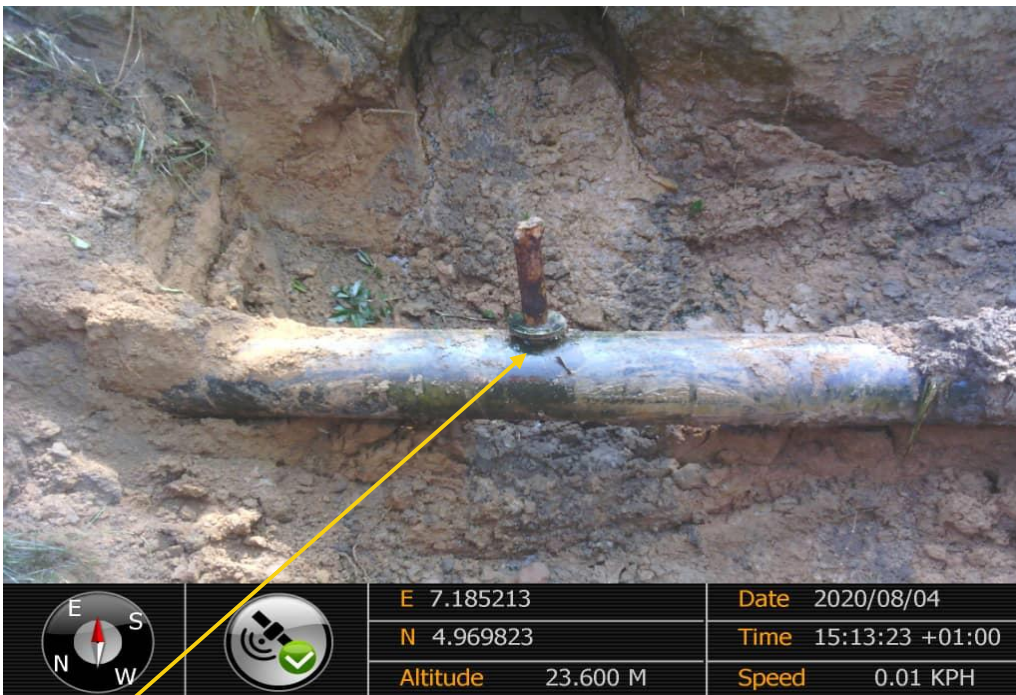
Close-up: 3" Welded Neck Flange installed at 12 o'clock position on 12" ImoRiver2 - Ogale Pipeline at Umulolo. Picture was taken during Joint Investigation 4 th August 2020.
