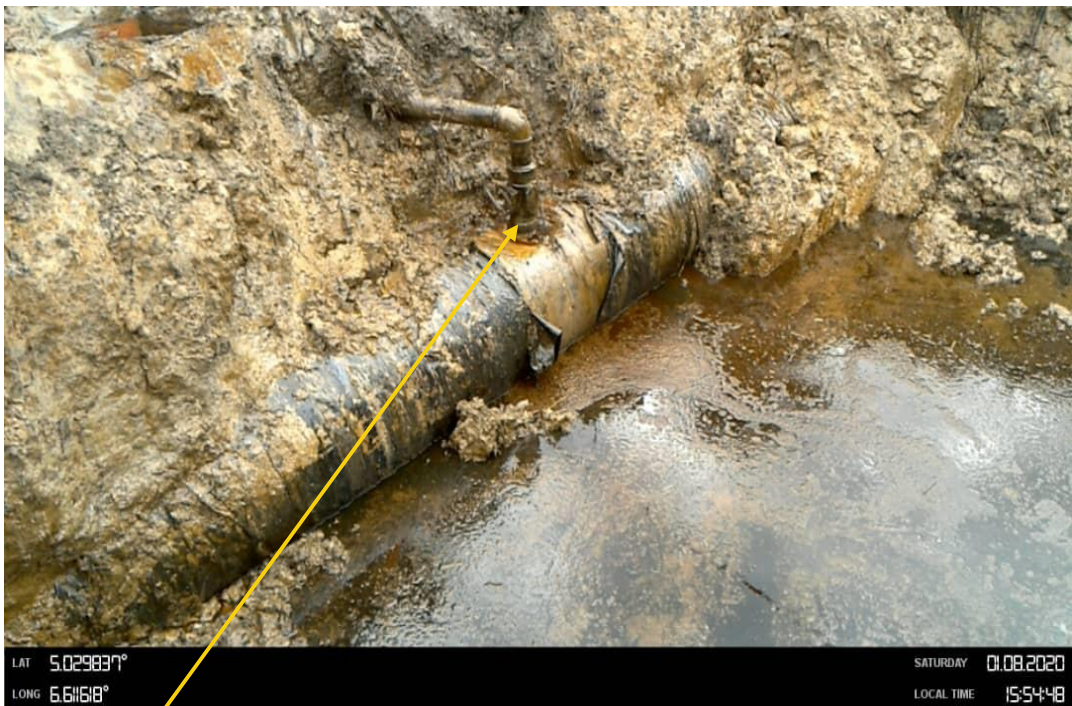
Close-up: 2" gate valve and 2" galvanized pipe installed at 12 o'clock position on 14" Okordia Rumuekpe Pipeline at Edeoha. Picture was taken during Joint Investigation on 1st August 2020.
