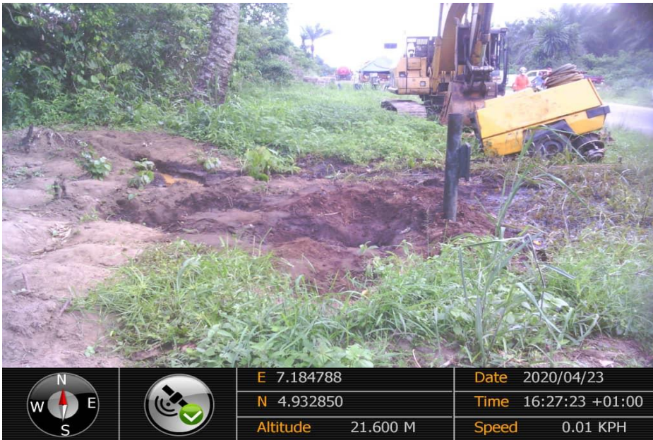
Overview: Part of spill impact on 12" Imo River 1- Ogale Pipeline at Etituzo-Umuololo . Picture was taken during Joint Investigation of 23 rd April 2020.
