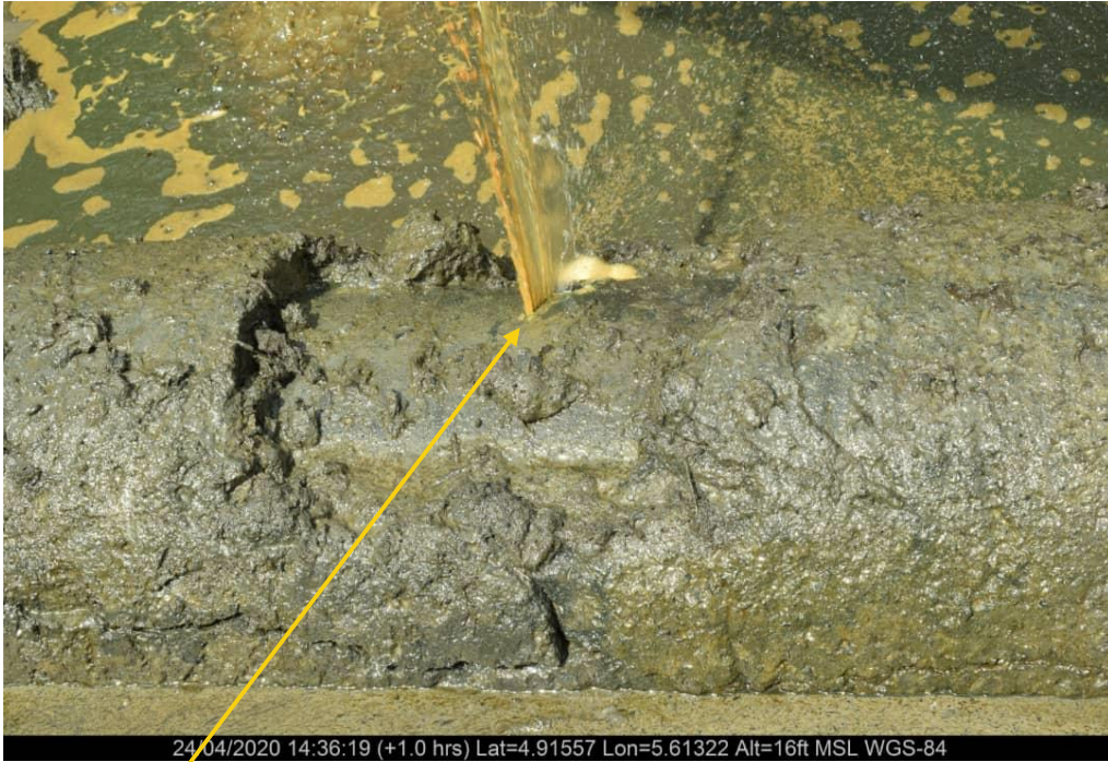
Close-up: Hack Saw Cut at 1 o'clock position on 16" Tunu – Brasscreek Pipeline at Agbidiana. Picture was taken during Joint Investigation of 24 th April 2020.
