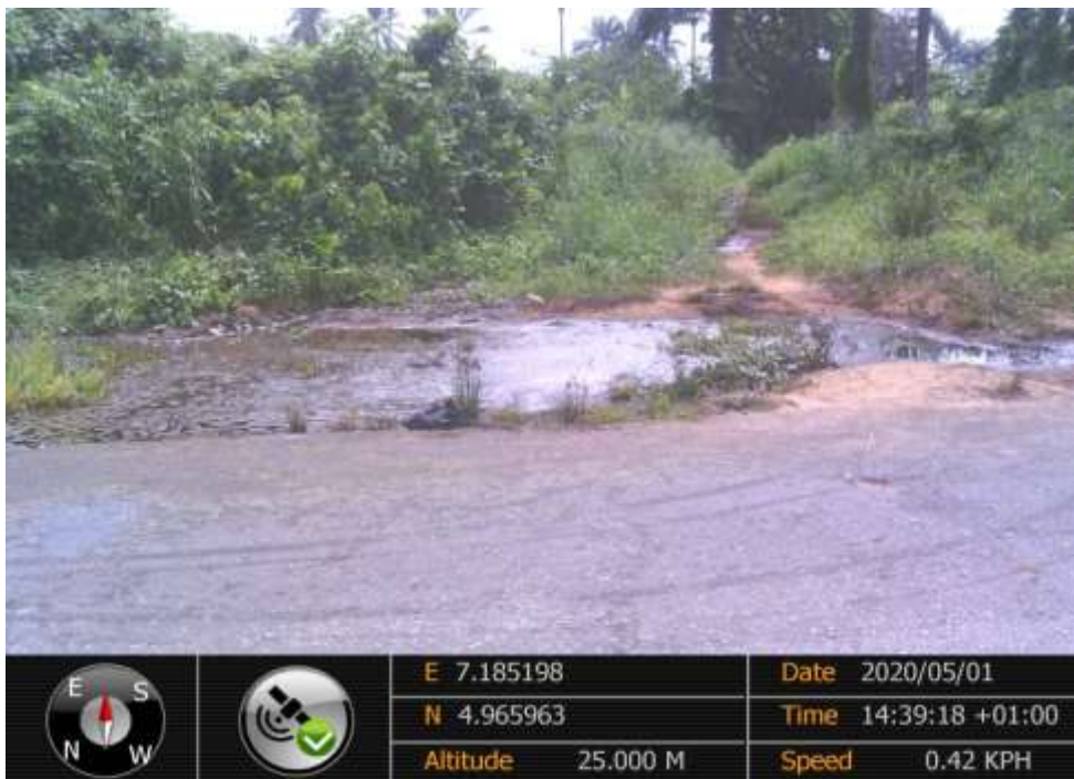
Overview: Part of spill impact on 12" ImoRiver 2 – Ogale Pipeline at Umulolo. Picture was taken during Joint Investigation 1st May 2020.
