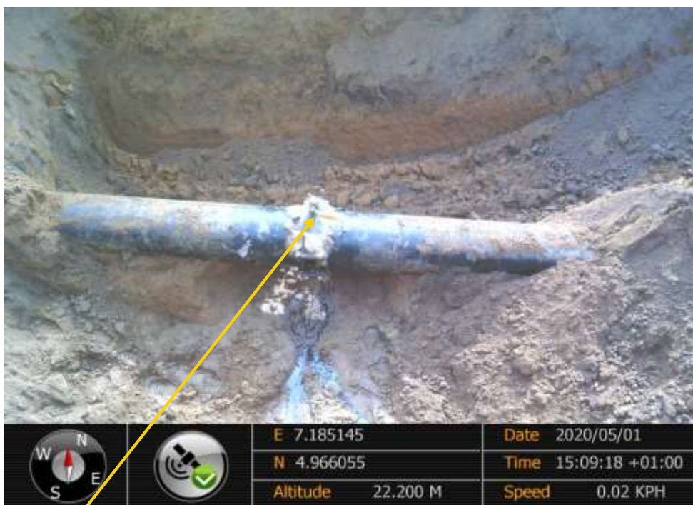
Close-up: Crude oil theft point installed at 12 o'clock position on 12" ImoRiver 2 Ogale Pipeline at Umulolo. Picture was taken during Joint Investigation 1st May 2020.
