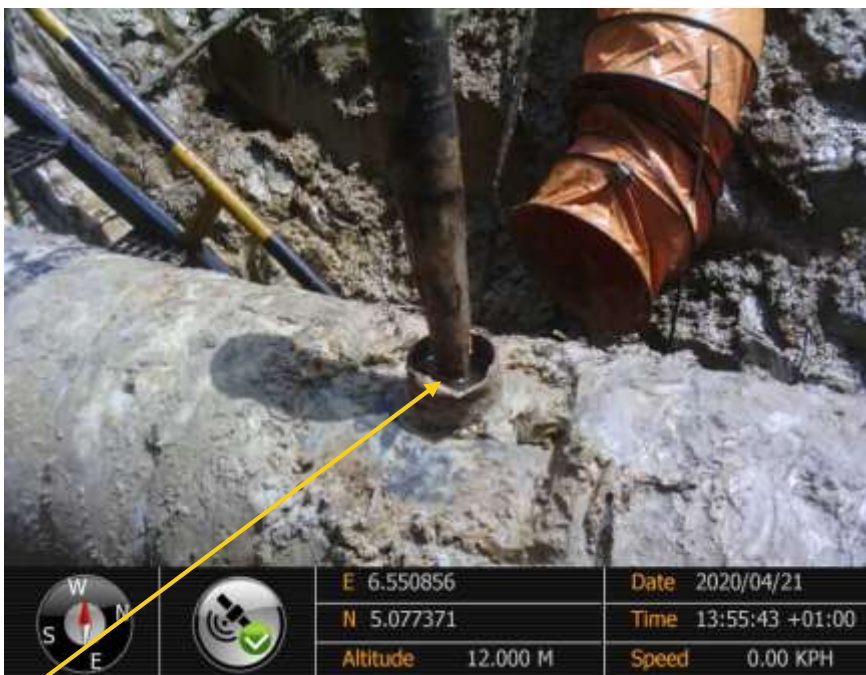
Close-up: 3" Nipple Installed at 12 o'clock position on Picture was taken during Joint Investigation of 21 st April 2020.
