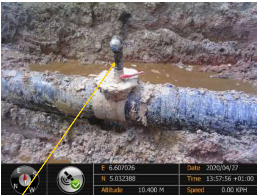
Close-up: 3" Valve Installed at 12 o'clock position on 14" Okordia Rumuekpe Pipeline at Edeoha. Picture was taken during Joint Investigation of 27 th April 2020.
