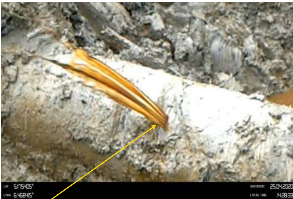
Close-up: 15mm Hacksaw cut at 11 o'clock position on 12" Adibawa Okordia Pipeline at Ikarama. Picture was taken during Joint Investigation of 25 th April 2020.
