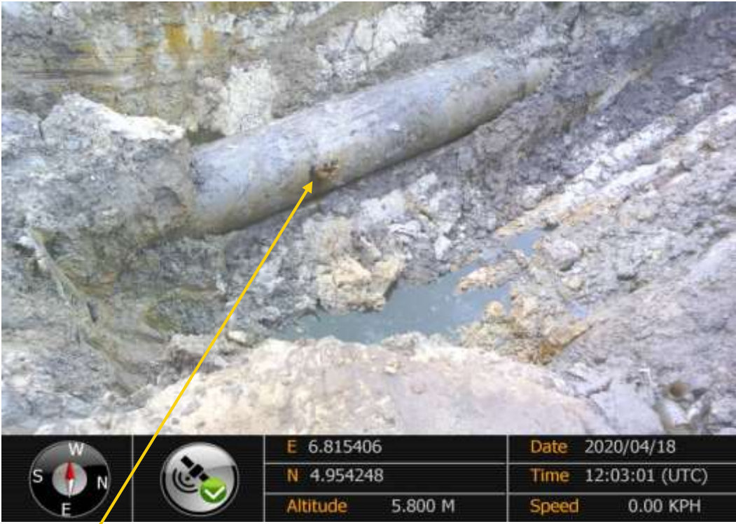
Close-up: 10mm drilled hole at 3 o'clock position on 20" Rumuekpe Nkpoku Pipeline at Ibaa. Picture was taken during Joint Investigation of 18 th April 2020.
