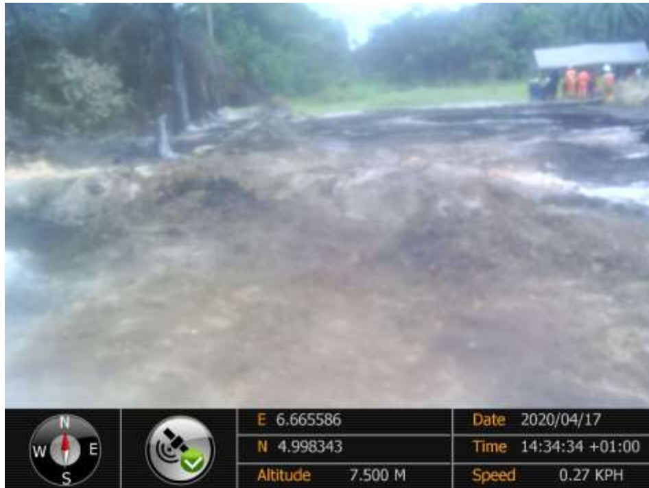
Overview: Part of spill impact on 14" Okordia – Rumuekpe Pipeline at Ihunwo. Picture was taken during Joint Investigation of 17 th April 2020.
