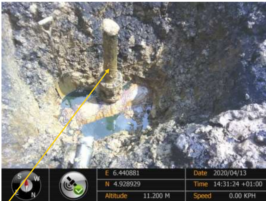
Close-up: 4" ball valve flange installed at 12 o'clock position on 20" Kolocreek - Rumuekpe pipeline at Odau KP 9.4 . Picture was taken during Joint Investigation of 13 th April 2020.
