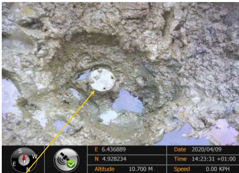
Close-up: Failed 3” theft fittings installed at 12 o’clock position on 20” Kolocreek Rumuekpe Pipeline at Odau KP9. Picture was taken during Joint Investigation of 9 th April 2020.
