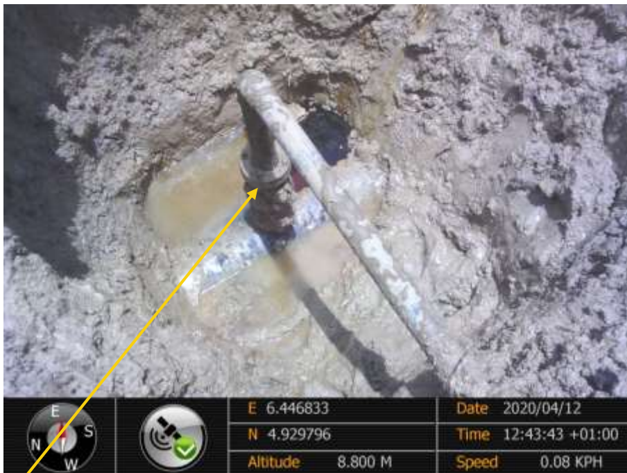
Close-up: 3" ball valve flange installed at 12 o'clock position on 20" Kolocreek – Rumuekpe Pipeline at Odau KM10. Picture was taken during Joint Investigation of 12 th April 2020.
