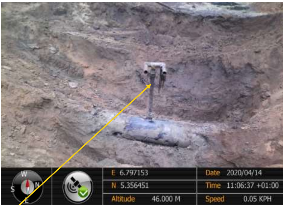
Close-up: Crude oil theft point at 12 o'clock position on 18" Assa Rumuekpe Pipeline at Ochia-Awara. Picture was taken during Joint Investigation of 14 th April 2020
