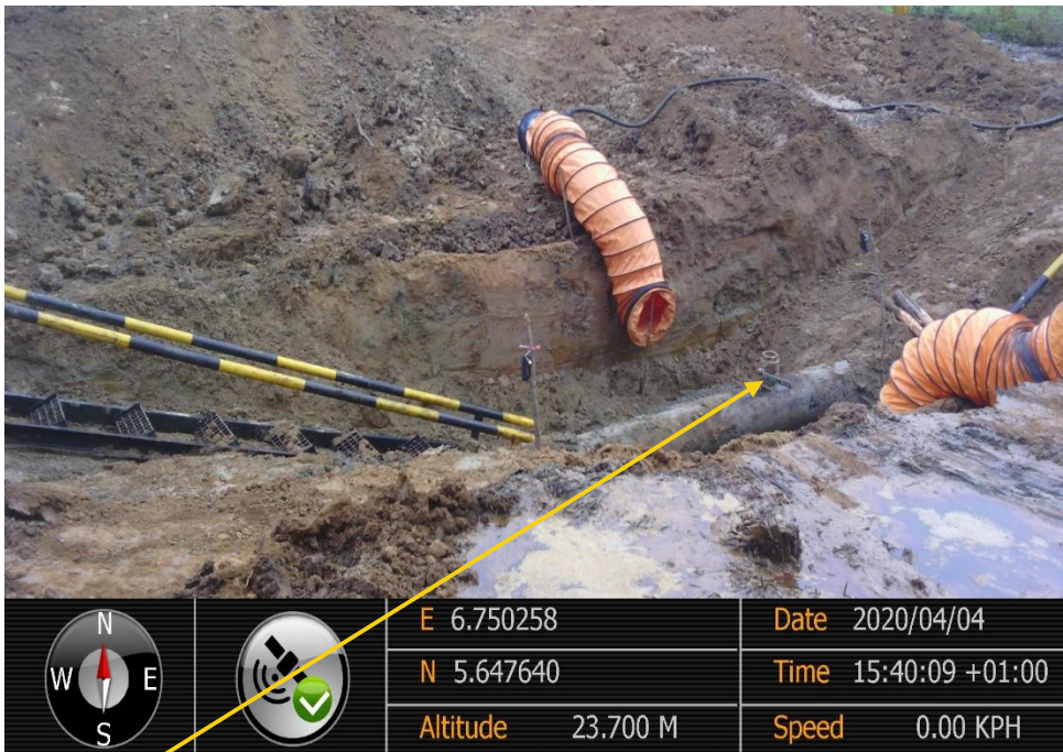
Close-up: 4" valve installed at 12 o'clock position on 12" Oguta – Egbama Pipeline at Umunkwu. Picture was taken during Joint Investigation of 4 th April 2020.
