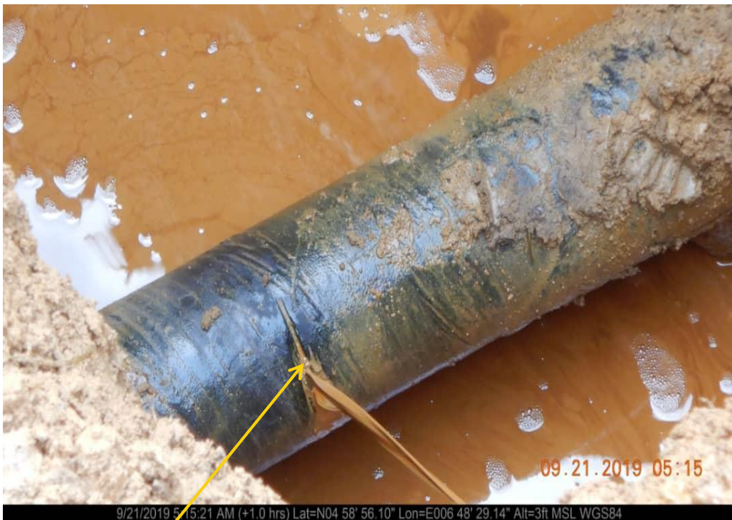
Close-up: Hacksaw Cut on 4" Obelle - Ibaa Pipeline at Ibaa. Picture was taken during Joint Investigation of 21 st September 2019.
