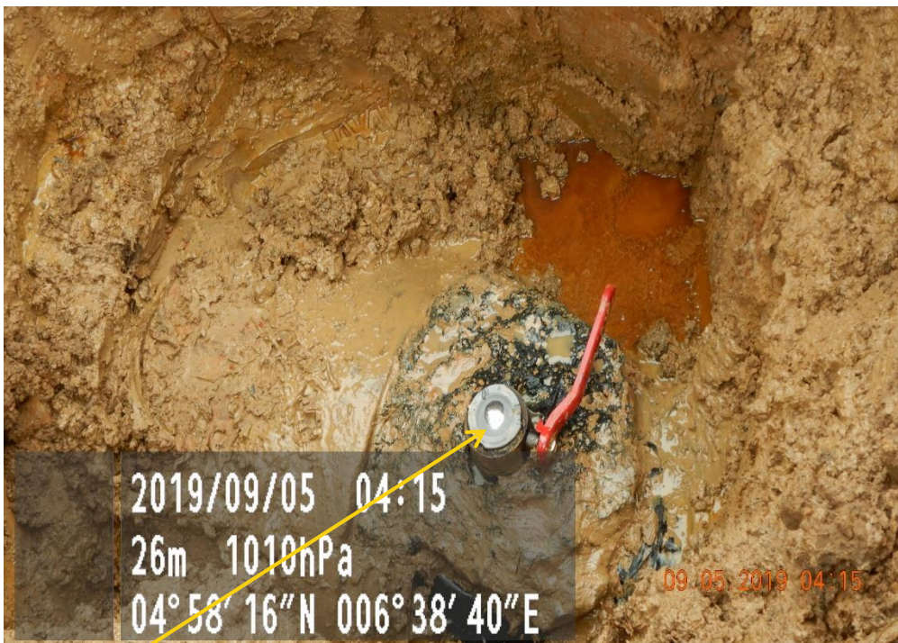
Close-up: Illegal fitting on New 20" Kolocreek - Rumuekpe Pipeline at Okoma1. Picture was taken during Joint Investigation of 5 th September 2019.
