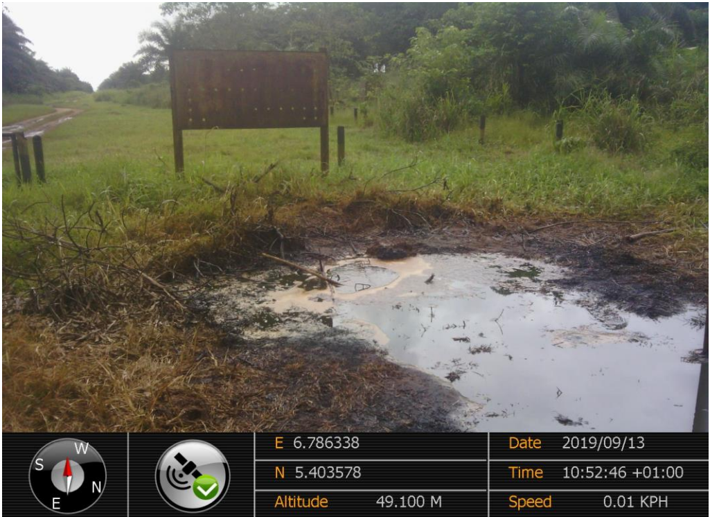
Overview: Part of spill impact on 16" Egbema – Assa Pipeline Right of Way at Obile. Picture was taken during Joint Investigation of 13 th September 2019.
