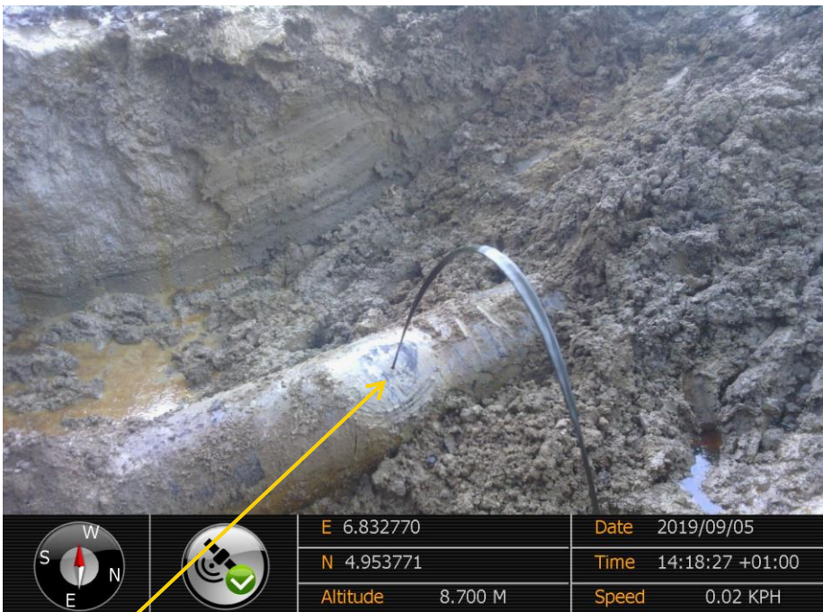
Close-up: Drilled Hole on 20'' Rumuekpe - Nkpoku Pipeline at Ibaa. Picture was taken during Joint Investigation of 5 th September 2019.
