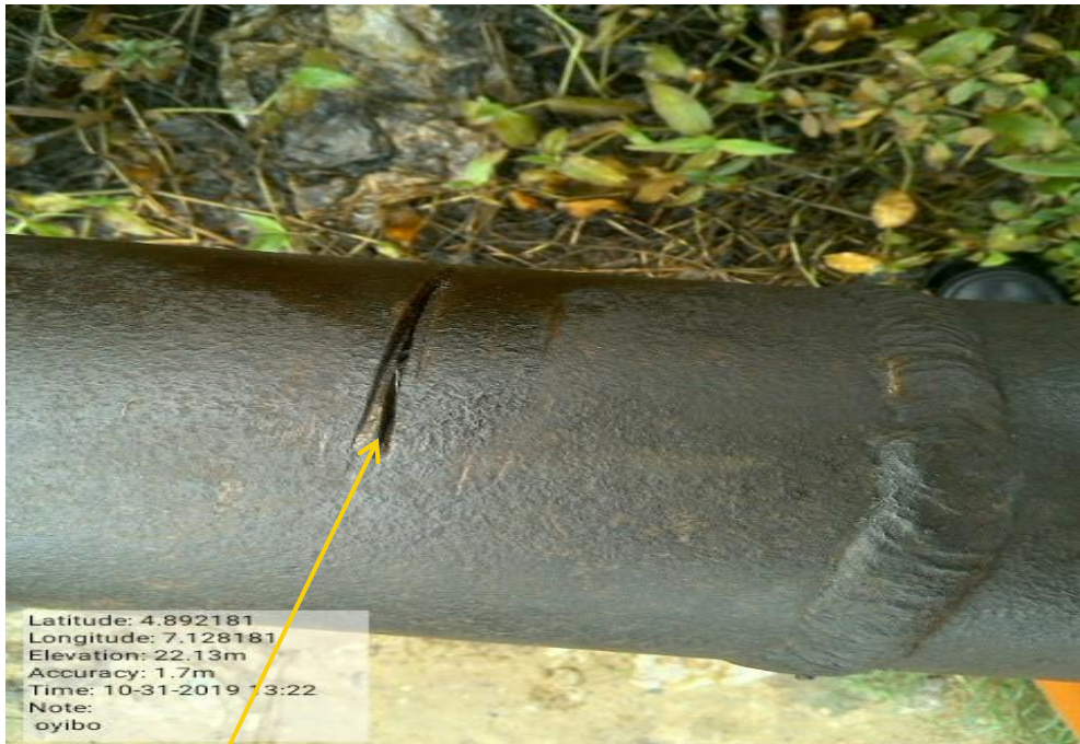
Close-up: Hack Saw Cut on 4" Obigbo Well 38 & 52 Flowline at Umuebulu. Picture was taken during Joint Investigation of 31 st October 2019.
