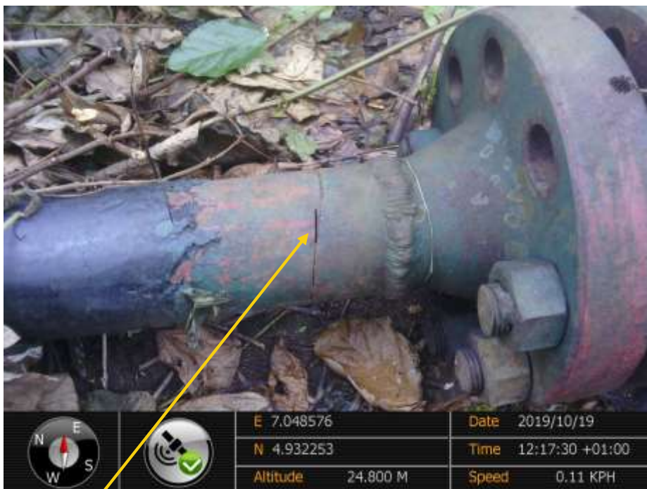
Close-up: hacksaw cut on Agbada 2 well 62L Flowline at Omueke. Picture was taken during Joint Investigation of 19 th October 2019.
