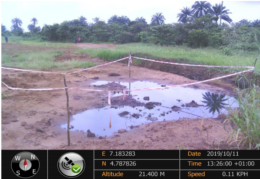
Overview: Part of spill impact on 24" Nkpoku - Bomu Pipeline Right of Way at Egbalor. Picture was taken during Joint Investigation of 11 th October 2019.
