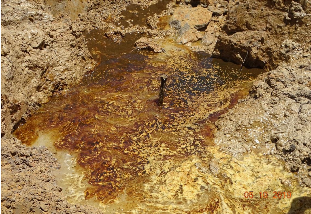
Overview: Part of spill impact on 14" Okordia - Rumuekpe Pipeline Right of Way at Ikata Picture was taken during Joint Investigation of 5 th October 2019.
