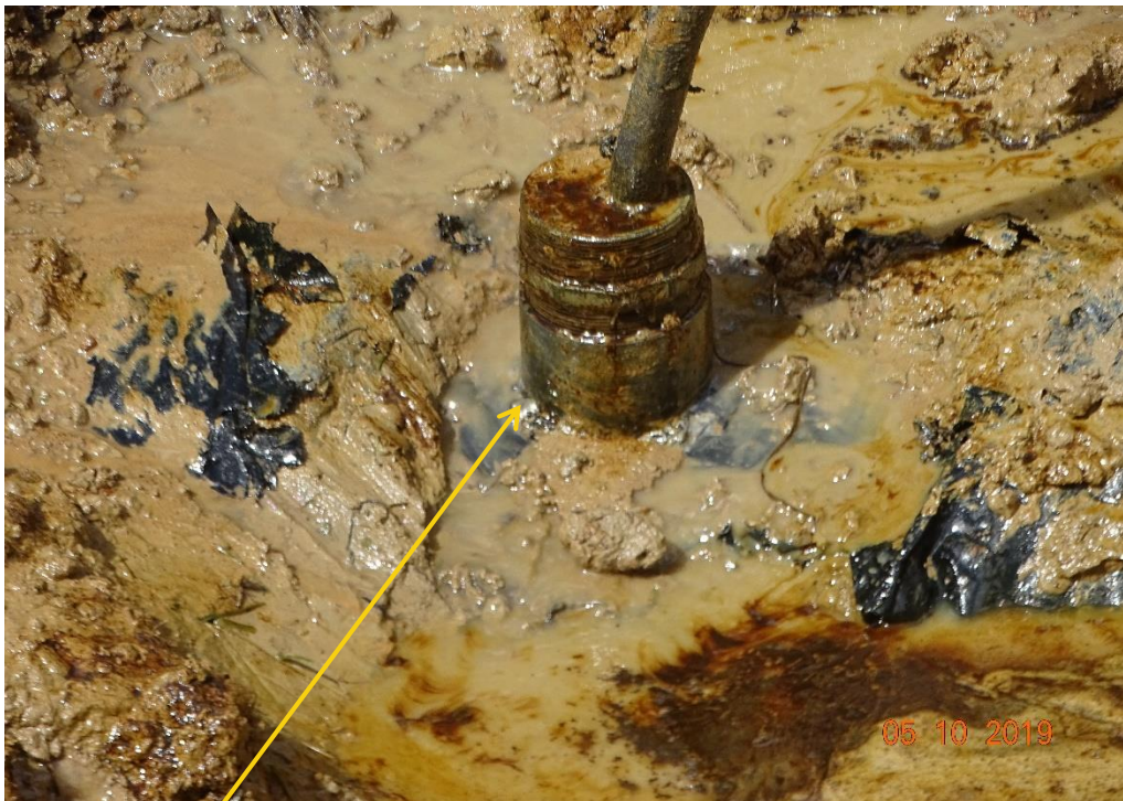
Close-up: Illegal fitting on 14" Okordia - Rumuekpe Pipeline at Ikata. Picture was taken during Joint Investigation of 5 th October 2019.
