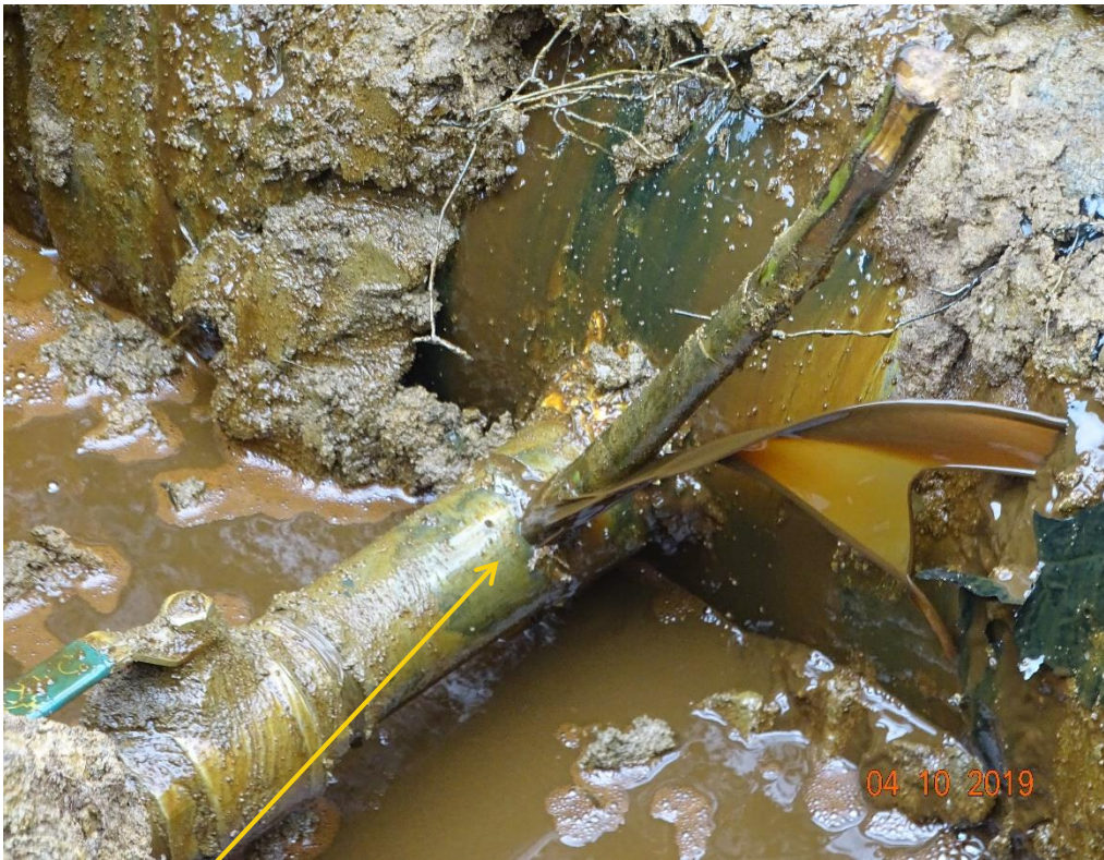
Close-up: Illegal fitting on 14" Okordia - Rumuekpe Pipeline at Ikata. Picture was taken during Joint Investigation of 4 th October 2019.
