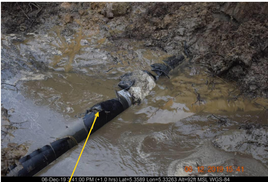
Close-up: Ruptured gas flowline on 6'' well 121T Flowline at Youbebe. Picture was taken during Joint Investigation of 6 th December 2019.
