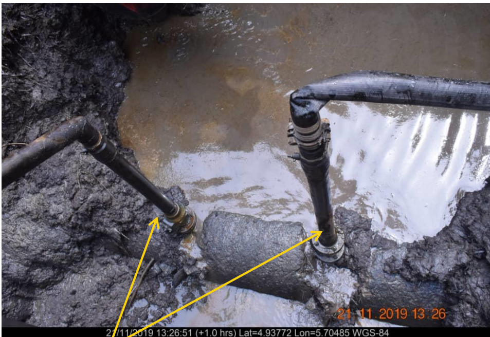
Close-up: Illegal Fittings on 20 " Opukushi - Brasscreek at Tamogbene. Picture was taken during Joint Investigation of 21 st November2019
