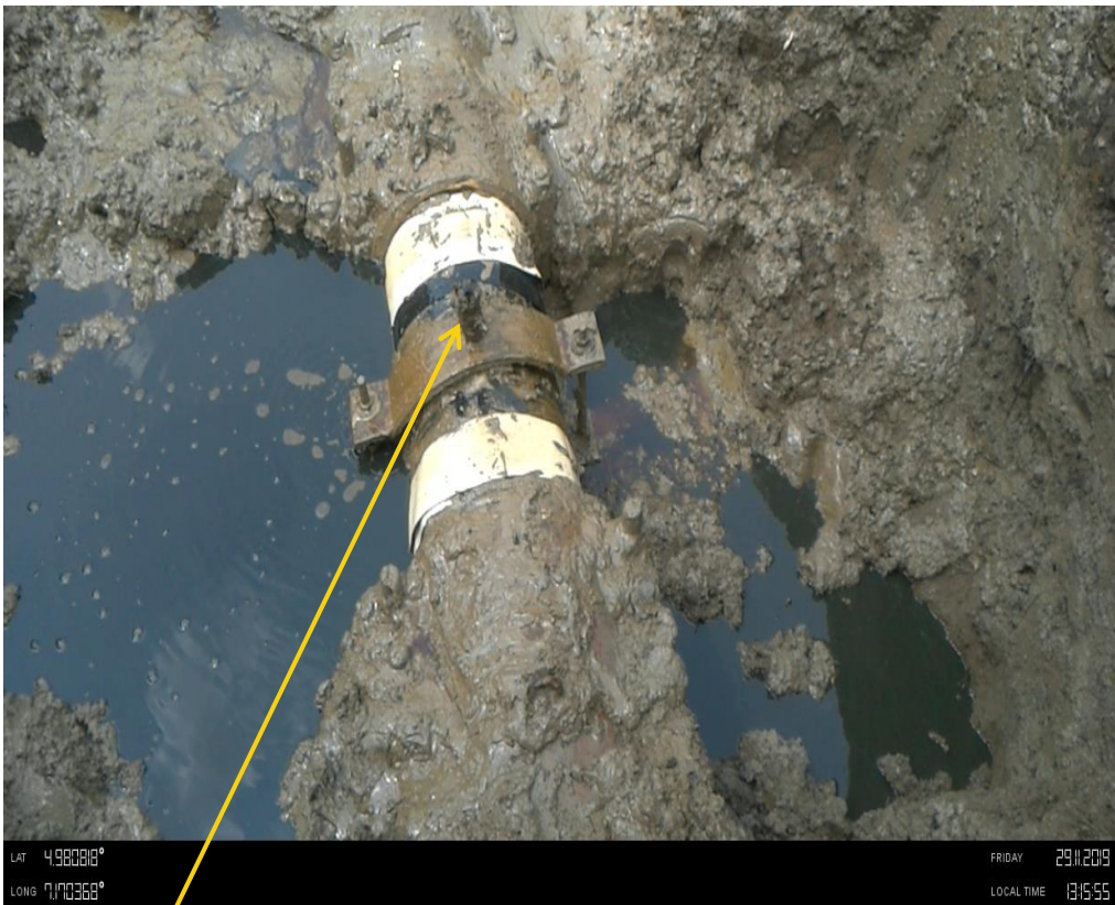
Close-up: Illegal fitting on 12'' Imo River2 – Ogale Pipeline at Odagwa . Picture was taken during Joint Investigation of 29 th November 2019.
