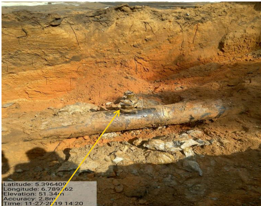
Close-up: Illegal Fitting on 16'' Egbema – Assa Pipeline at Obile. Picture was taken during Joint Investigation of 27 th November 2019.
