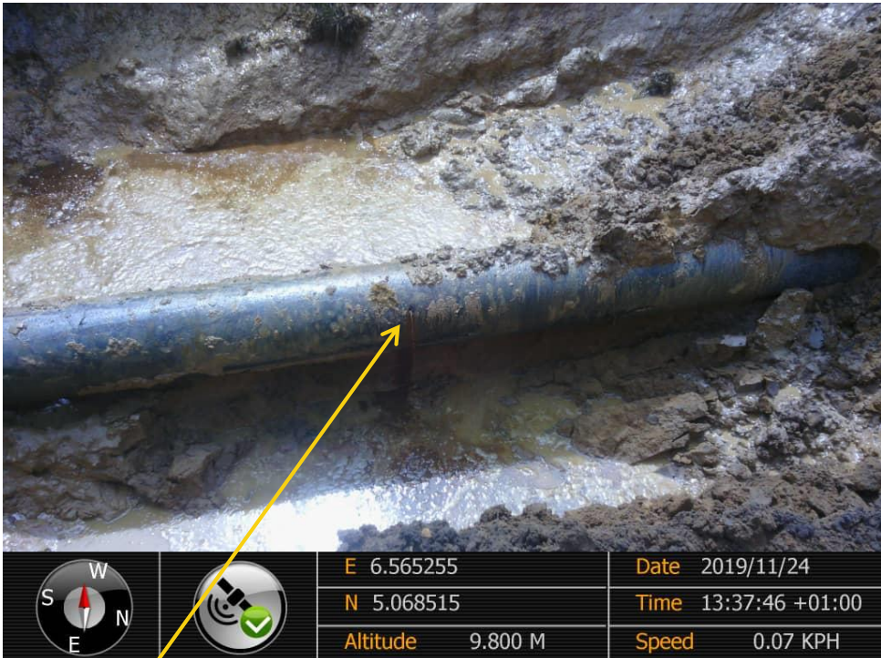
Close-up: Drilled Hole on 14" Okordia – Rumuekpe Pipeline at Ula-Okobo . Picture was taken during Joint Investigation of 24 th November 2019.
