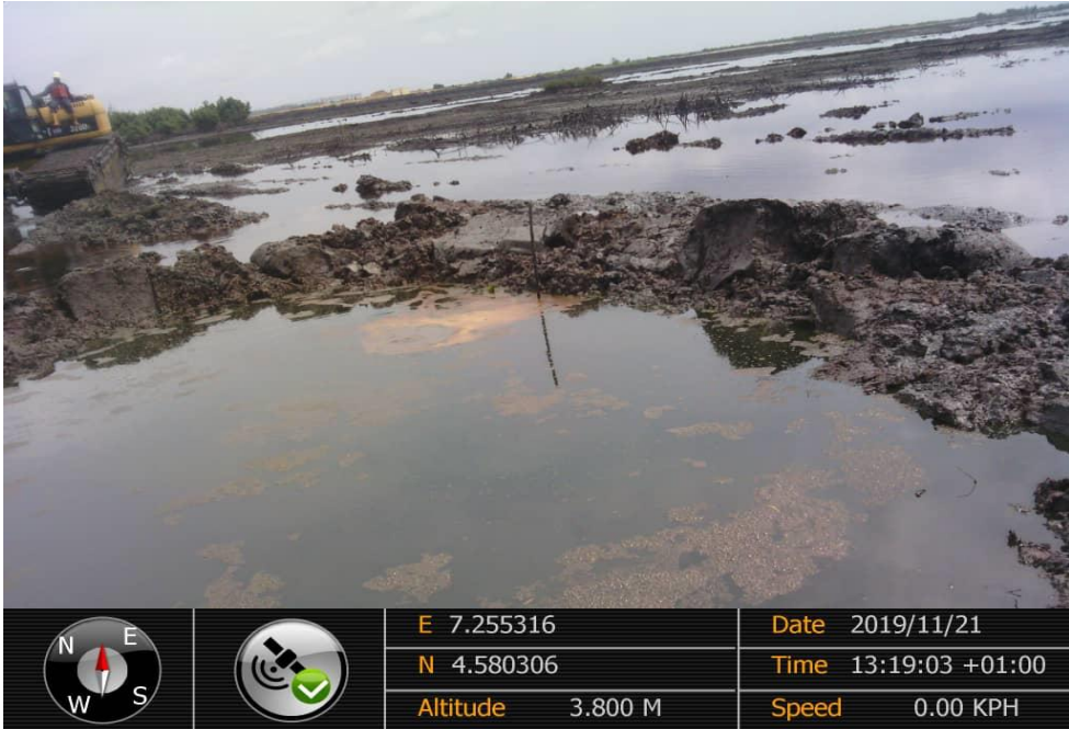
Overview: Part of spill impact on 28" Bomu – Bonny Pipeline Right of Way at Patrick Waterside - Bodo West . Picture was taken during Joint Investigation of 21 st November 2019.
