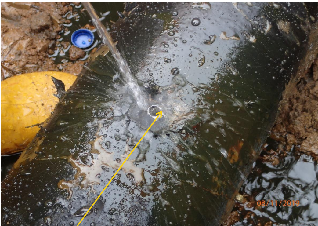
Close-up: Drilled Hole on 8" Isimiri – Imogate Pipeline at Uzuaku. Picture was taken during Joint Investigation of 8 th November 2019.
