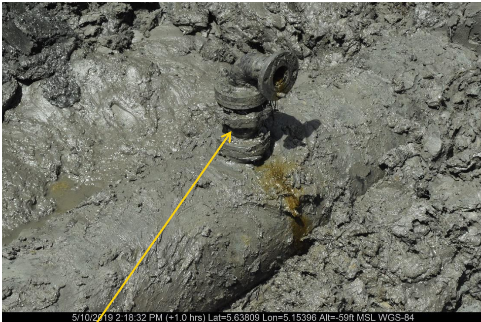
Close-up: Illegal fitting on 20" Otumara - escravos Pipeline at Ugboegungun. Picture was taken during Joint Investigation of 10 th May 2019.
