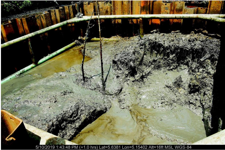
Overview: Part of spill impact on 20" Otumara - escravos Pipeline Right of Way at Ugboegungun. Picture was taken during Joint Investigation of 10 th May 2019.
