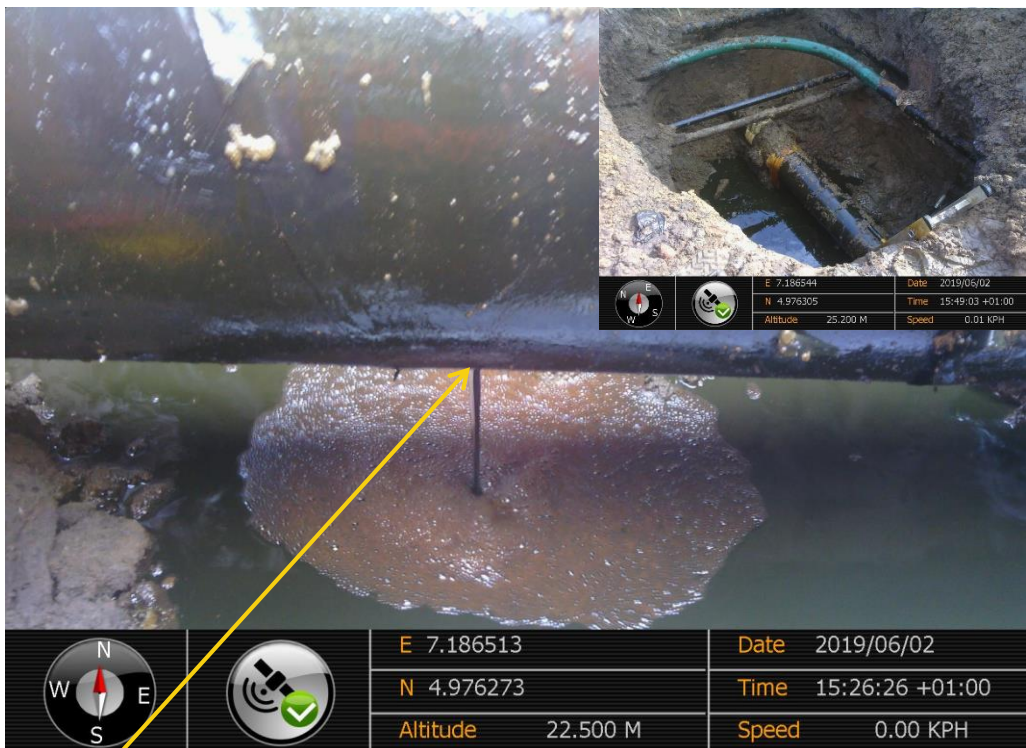
Close-up: Corrosion on 12" Imo River – Ogale Pipeline at Igiriukwu-Owaza. Picture was taken during Joint Investigation of 2 nd June 2019.
