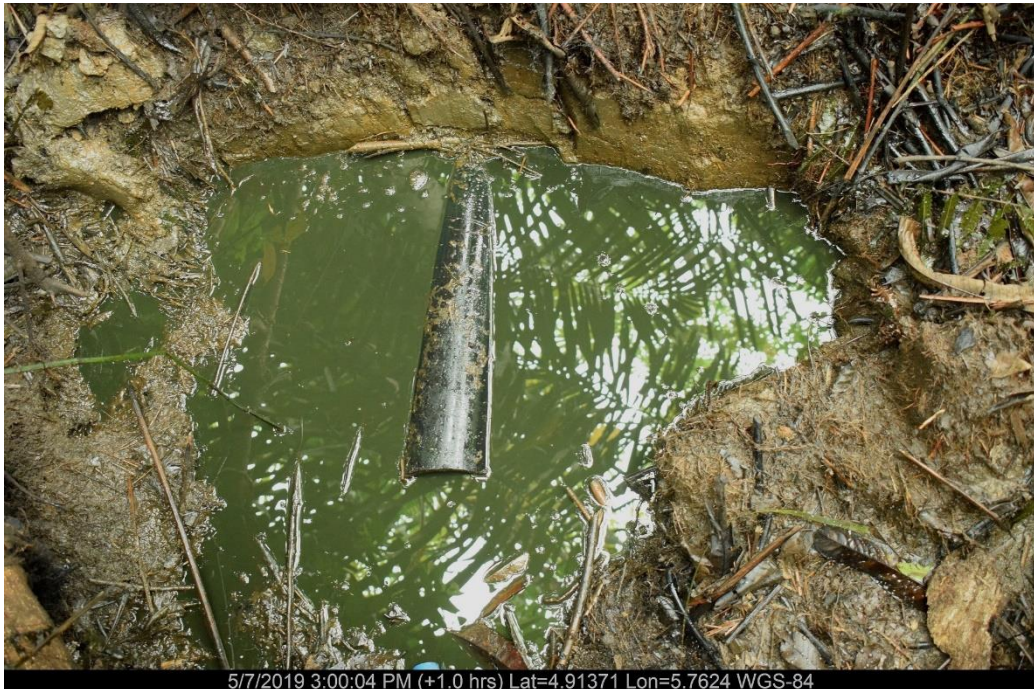
Overview: Part of spill impact on 4" Opukushi Well 24T Flowline at Egbemo Analabiri & Agbidiana. Picture was taken during Joint Investigation of 7 th May 2019.
