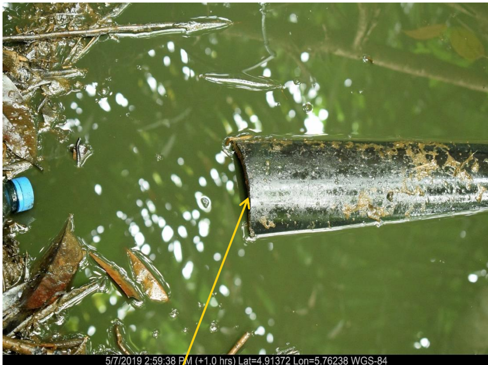
Close-up: Missing part of the Flowline on 4" Opukushi Well 24T Flowline at Egbemo Analabiri & Agbidiana. Picture was taken during Joint Investigation of 7 th May 2019.
