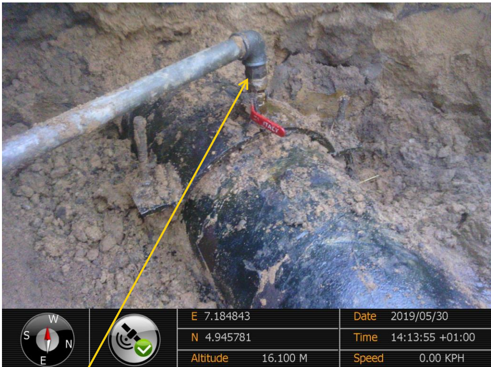
Close-up: Illegal fitting on 12" Imo River - Ogale Pipeline at Umuololo. Picture was taken during Joint Investigation of 30 th May 2019
