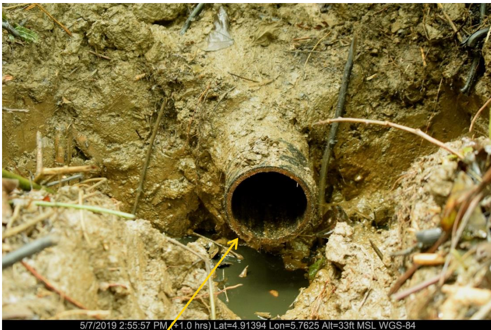
Close-up: Missing part of the Flowline on 4" Opukushi Well 9T Flowline at Egbemo-Analabiri-agbidiana. Picture was taken during Joint Investigation of 7 th May 2019.
