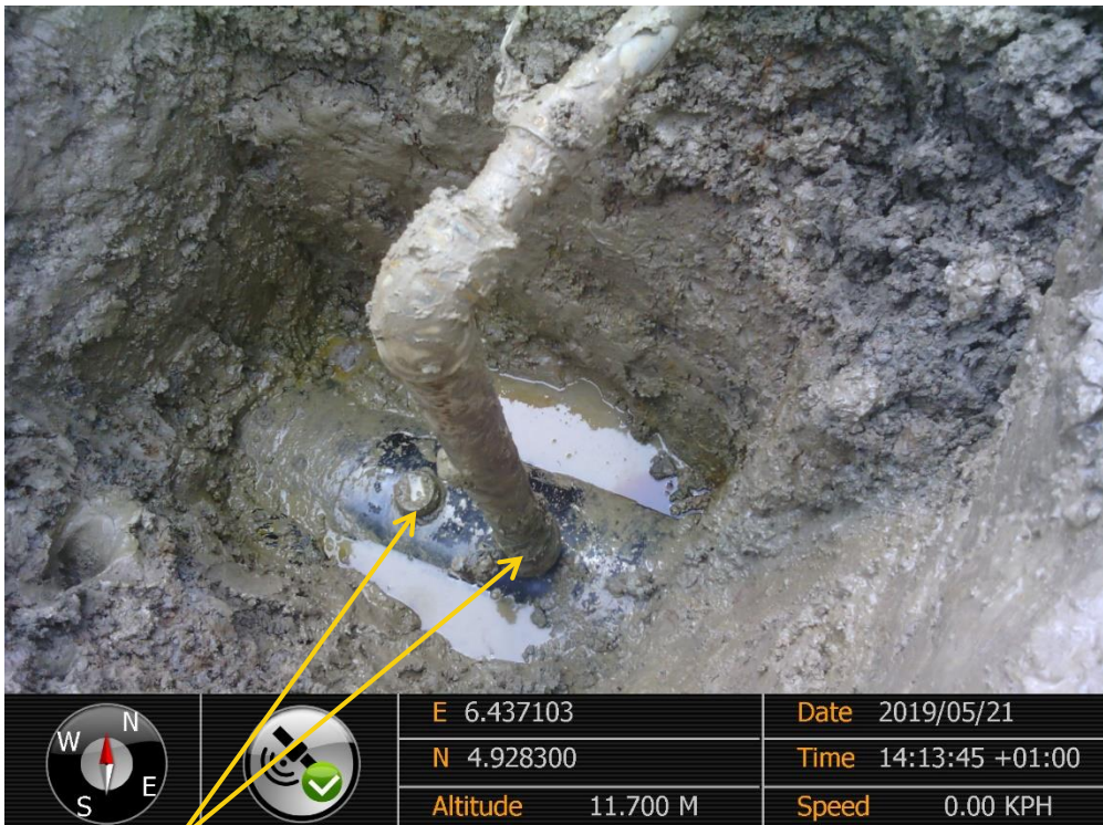
Close-up: Illegal fittings on 20'' Kolocreek – Rumuekpe Pipeline at Odau. Picture was taken during Joint Investigation of 21 st May 2019
