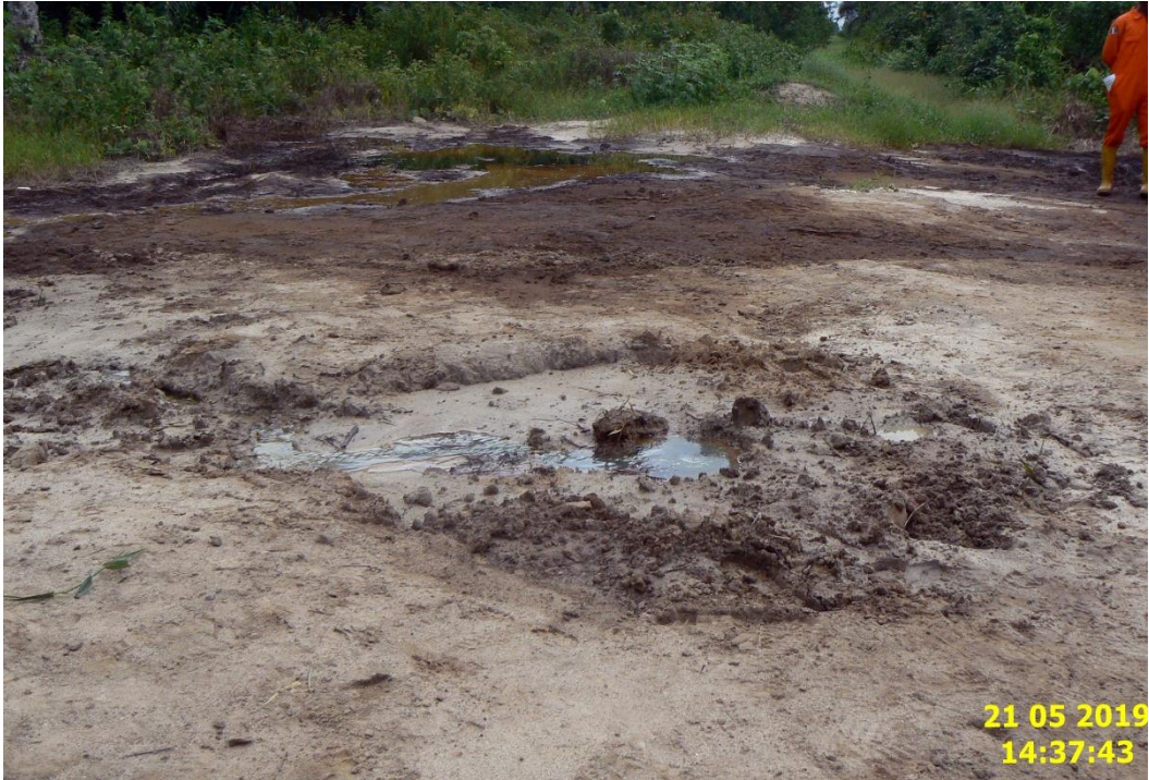
Overview: Part of spill impact on 20'' Kolocreek – Rumuekpe Pipeline Right of Way at Okoma-1. Picture was taken during Joint Investigation of 21 st May 2019.
