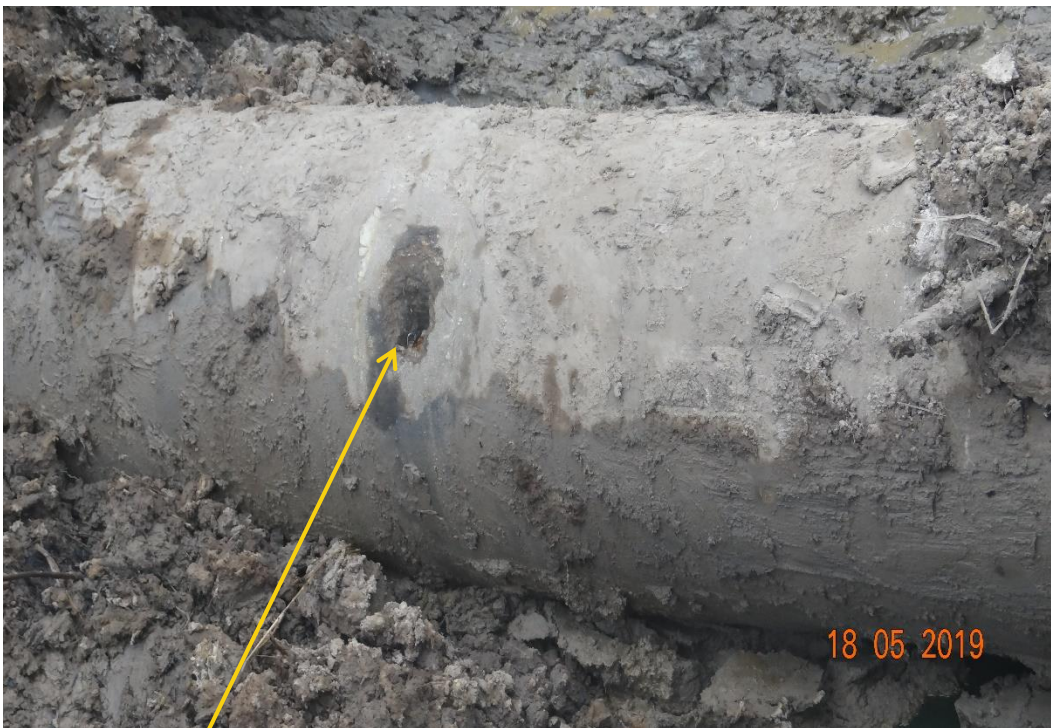
Close-up: Drilled Hole on 20" Kolocreek – Rumuekpe Pipeline at Okoma-1. Picture was taken during Joint Investigation of 18 th May 2019.
