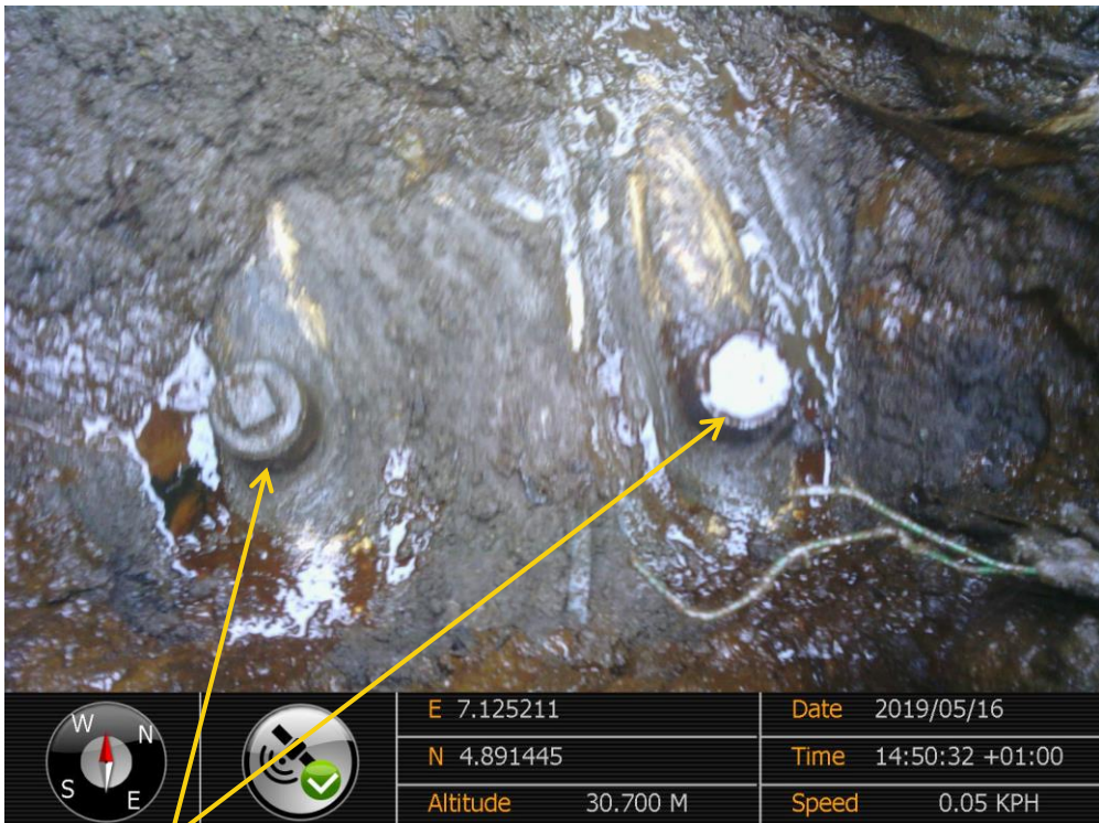
Close-up: Illegal Fittings on Obigbo North Well 3L/S Flowlines at Umuebulu. Picture was taken during Joint Investigation of 16 th May 2019
