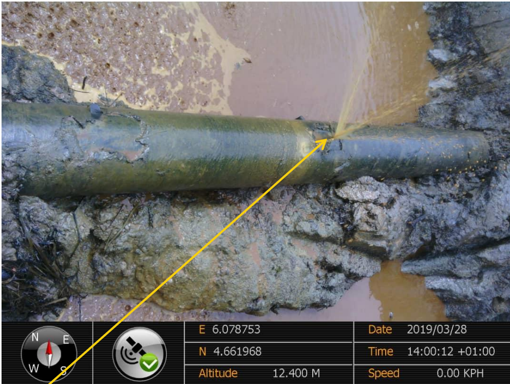
Close-up: Crack on 10'' Diebu Creek – Nun River Pipeline at Peremabiri. Picture was taken during Joint Investigation of 28 th March 2019
