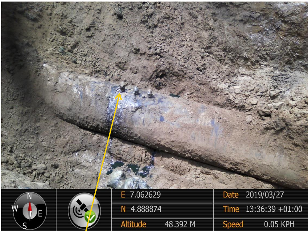
Close-up: Leaking Illegal fitting on 36'' Nkpoku - Bomu Pipeline at Atali. Picture was taken during Joint Investigation of 27 th March 2019
