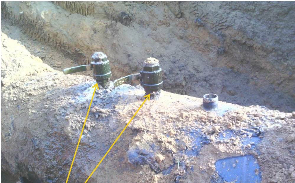
Overview: Part of spill impact on 28" Nkpoku - Bomu Pipeline Right of Way at Rumuowha-Eneka. Picture was taken during Joint Investigation of 29 th March 2019.
