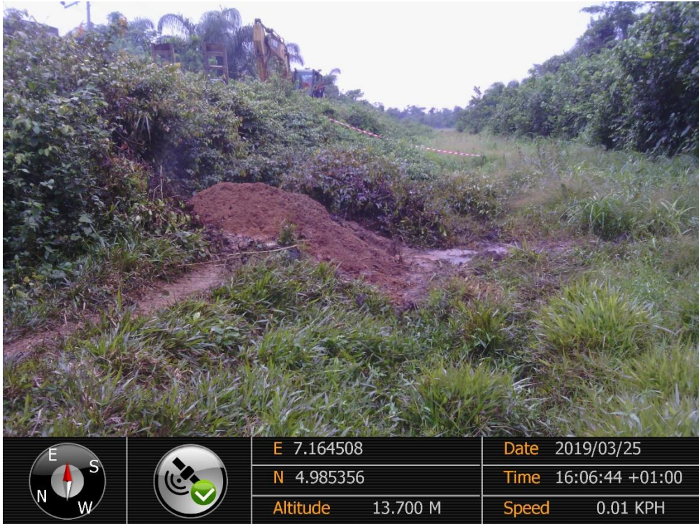
Overview: Part of spill impact on 8'' Nkali - ImoRiver Pipeline Right of Way at Odagwa. Picture was taken during Joint Investigation of 25 th March 2019.
