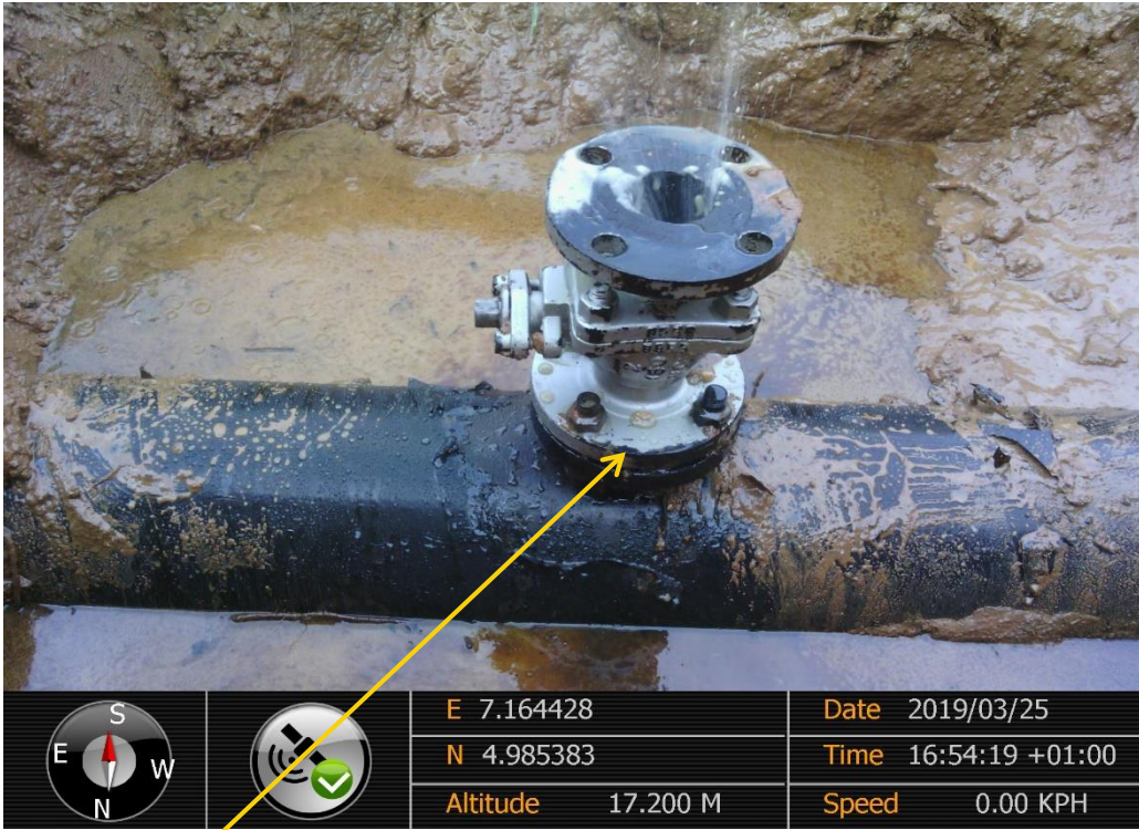
Close-up: Illegal Fitting on 8'' Nkali - ImoRiver Pipeline at Odagwa. Picture was taken during Joint Investigation of 25 th March 2019
