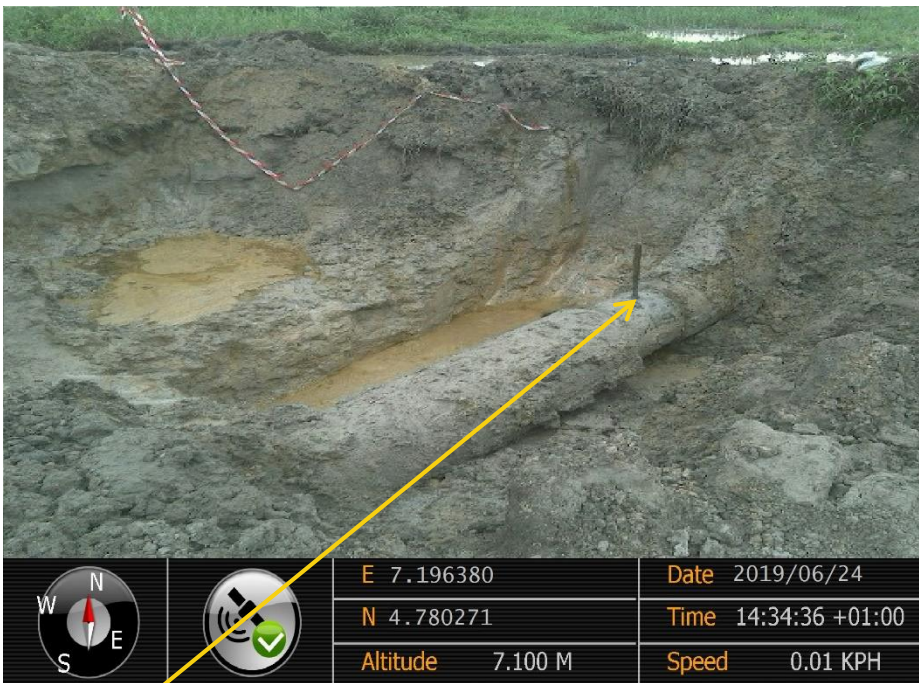
Close-up: Illegal Fitting on 24'' Nkpoku - Bomu Pipeline at Sime. Picture was taken during Joint Investigation of 24 th June 2019.
