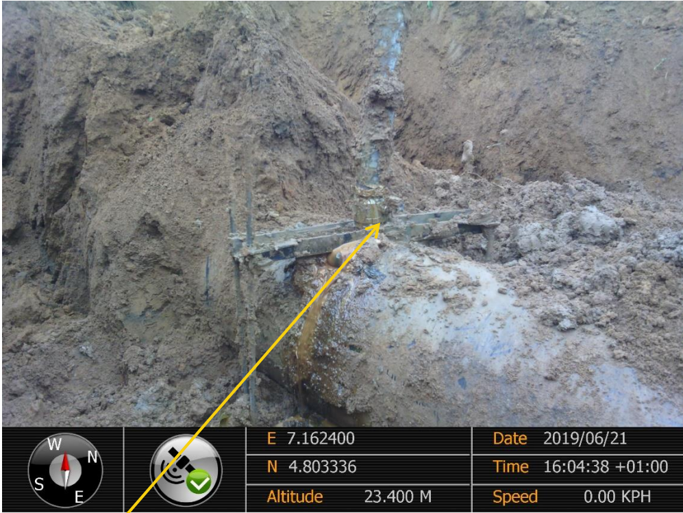
Close-up: Illegal Fitting on 24" Ogale – Bomu Pipeline at Agbeta. Picture was taken during Joint Investigation of 21 st June 2019.
