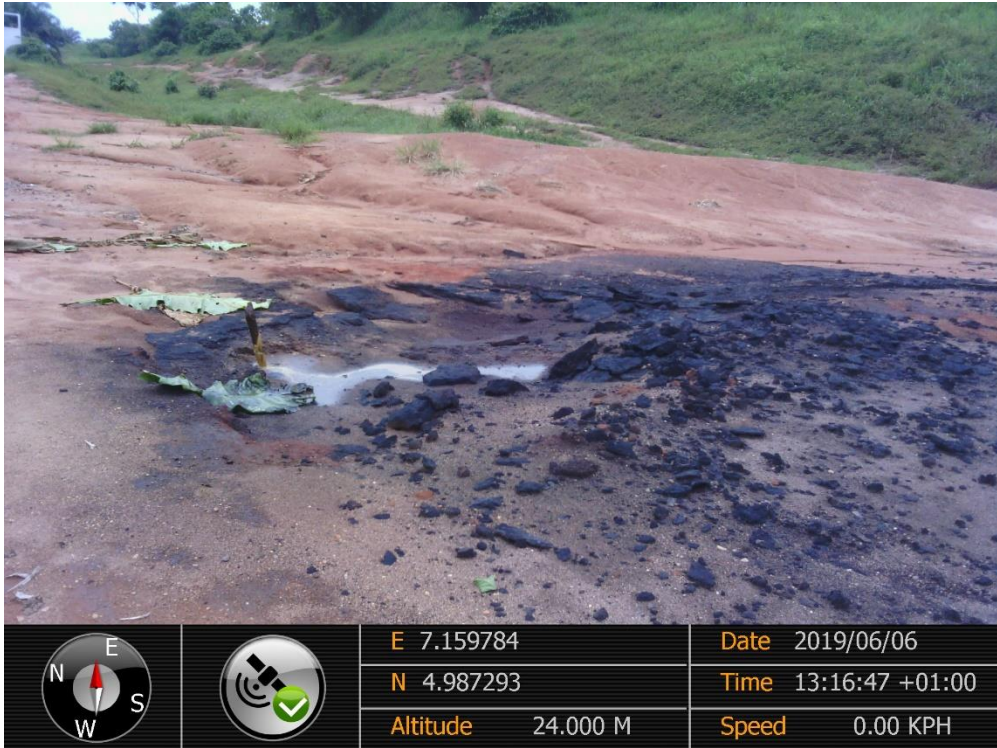
Overview: Part of spill impact on 8" Nkali – Imo River2 Pipeline Right of Way at Odagwa. Picture was taken during Joint Investigation of 6 th June 2019.
