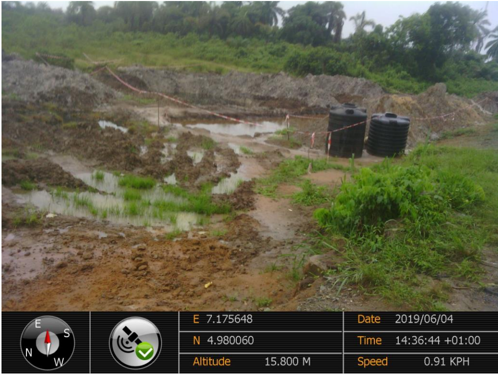
Overview: Part of spill impact on 12'' Imo River – Ogale Pipeline Right of Way at Owaza. Picture was taken during Joint Investigation of 4 th June 2019.
