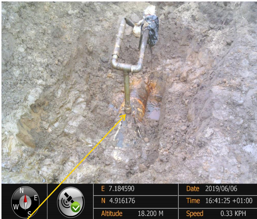
Close-up: Illegal fitting on 12" Imo River – Ogale Pipeline at Uzuaku. Picture was taken during Joint Investigation of 6 th June 2019
