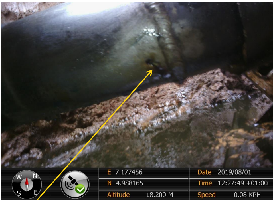
Close-up: Corrosion on Imo River Well 63T Flowline at Igiriukwu-Owaza. Picture was taken during Joint Investigation of 1 st August 2019.
